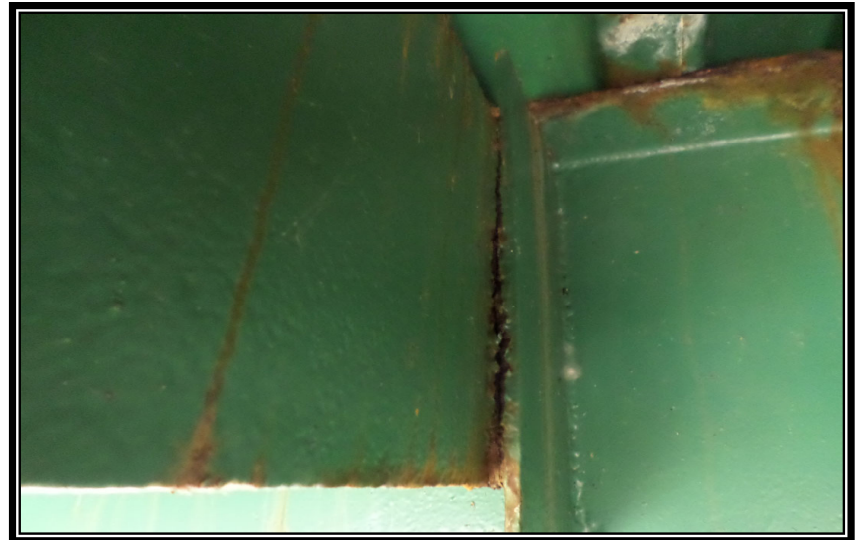
CRACKED VERTICAL DIAPHRAGM WELD
