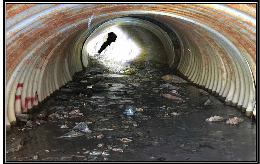
COLLAPSED CORRUGATED METAL PIPE CULVERT
