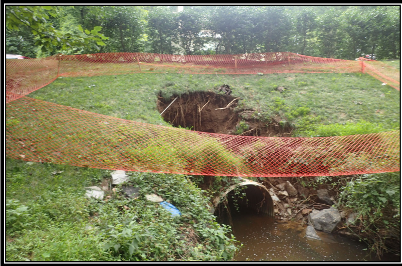
BEFORE CULVERT REAIRS
