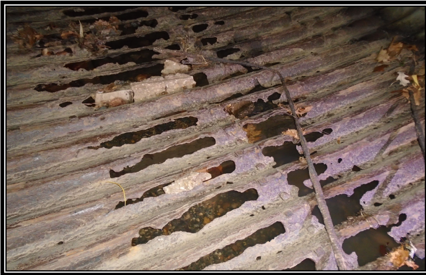
CORRUGATED METAL PIPE CULVERT SEVERE INVERT SECTION LOSS
