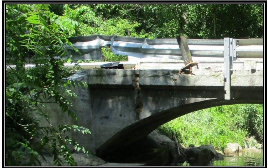
DAMAGED BRIDGE RAILING
