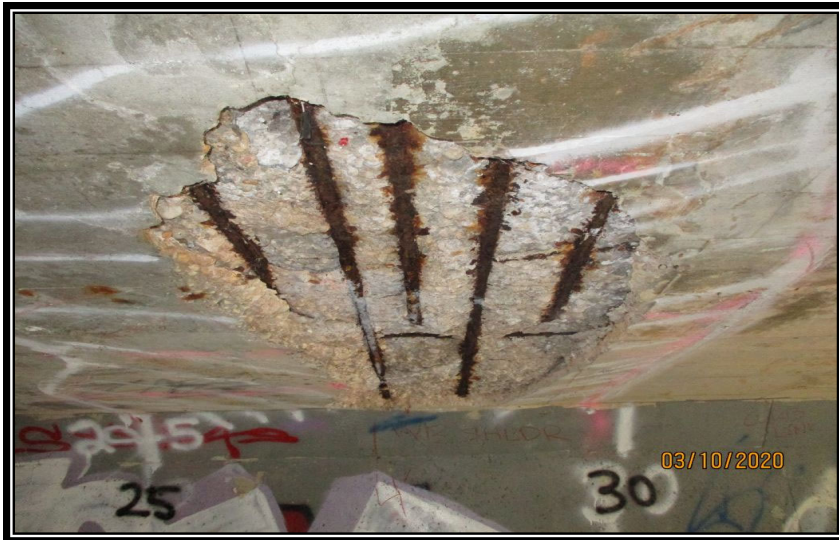
CONCRETE SPALLS WITH EXPOSED REINFORCING STEEL IN CULVERT TOP SLAB
