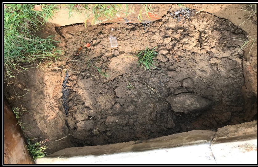
SINKHOLE ABOVE FAILED CORRUGATED METAL PIPE CULVERT
