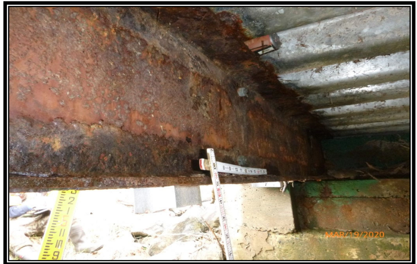
HEAVY RUST AND STEEL DELAMINATION
