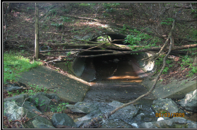
BEFORE CULVERT REPAIRS
